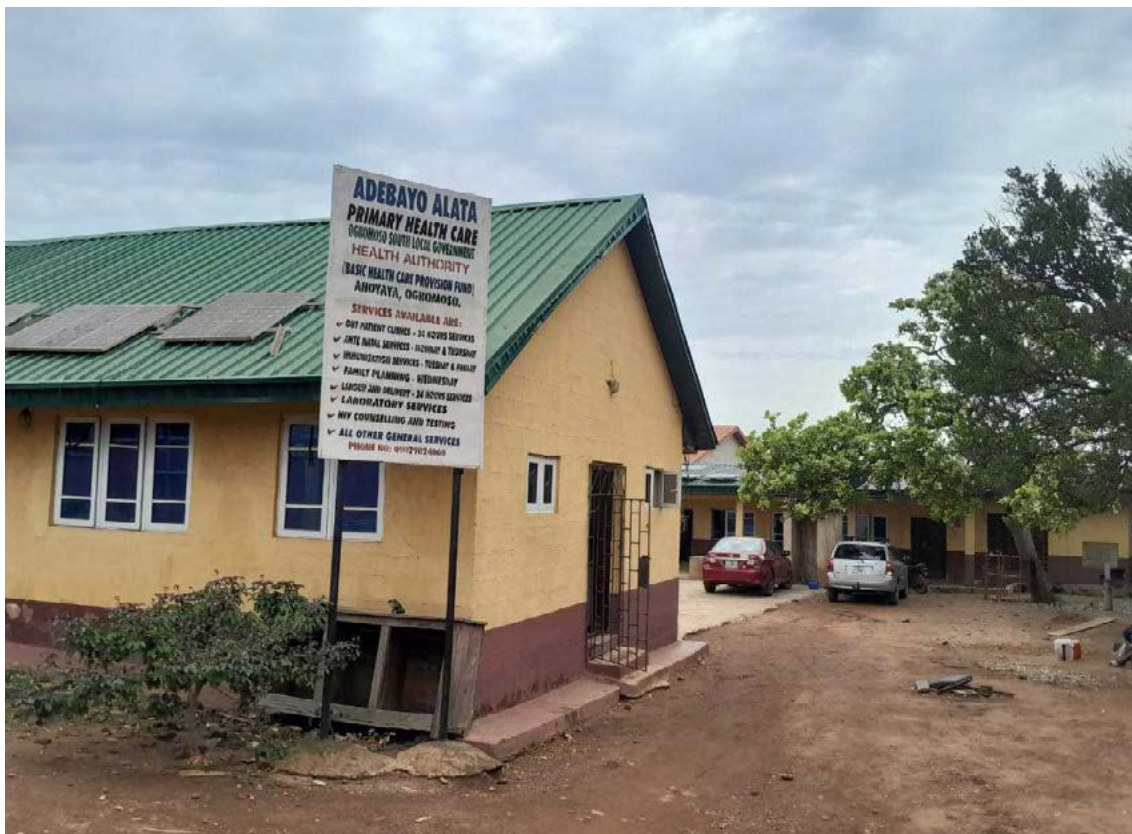
The Adebayo Alata Primary Health Care Centre in Ogbomosho, Nigeria, stands as a critical outpost for essential medical services in the community.
