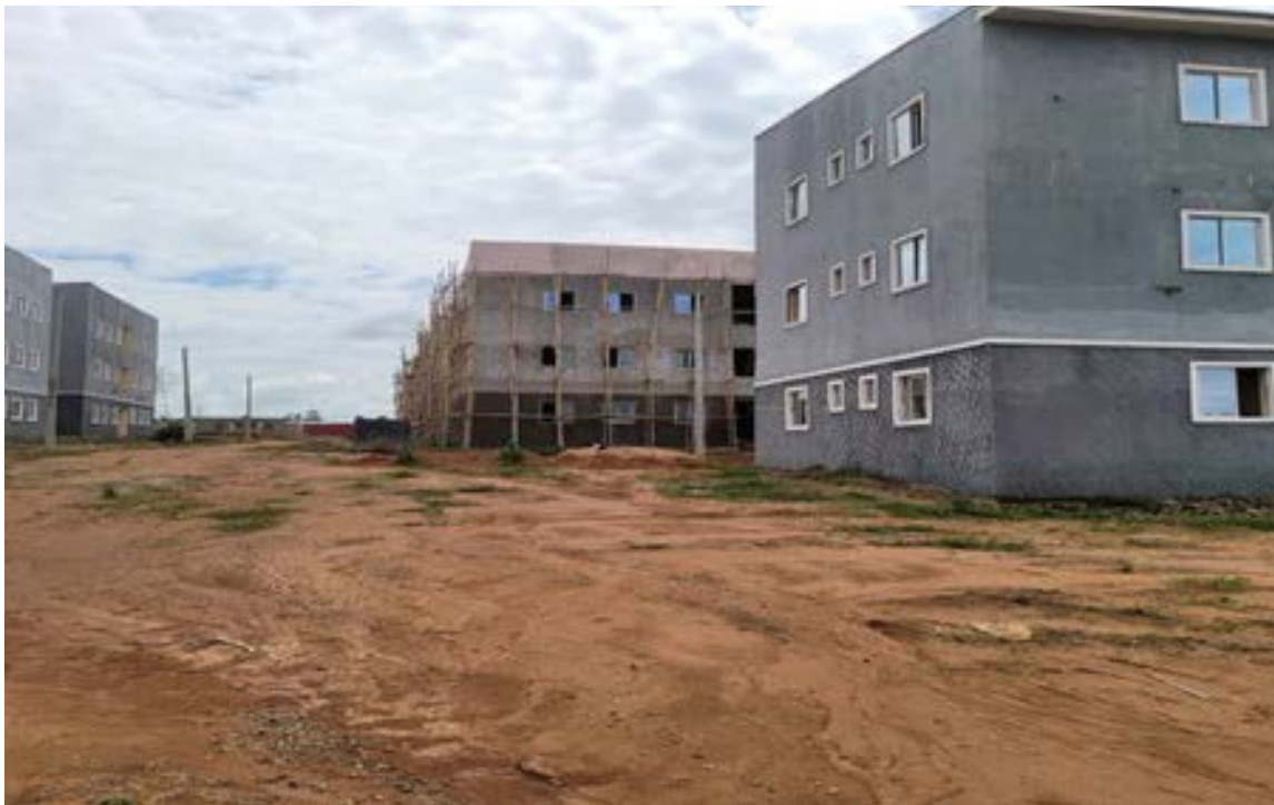
Caption: Wisar Estate, a Federal Mortgage Bank of Nigeria’s project under construction in Abuja
